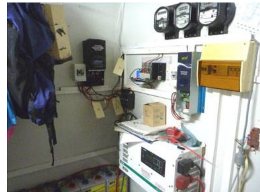
Power room at the Cape Tribulation research station. It also doubles as a laundry and clothing storage area.
