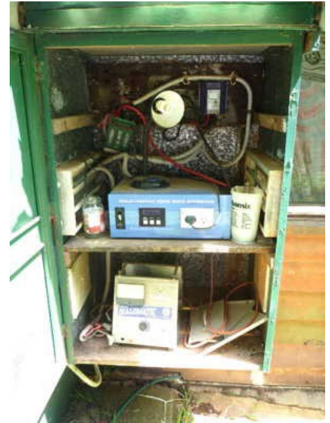
A post-1996 installation. There are still many of these in the Daintree! The battery box is to the left (not visible).
